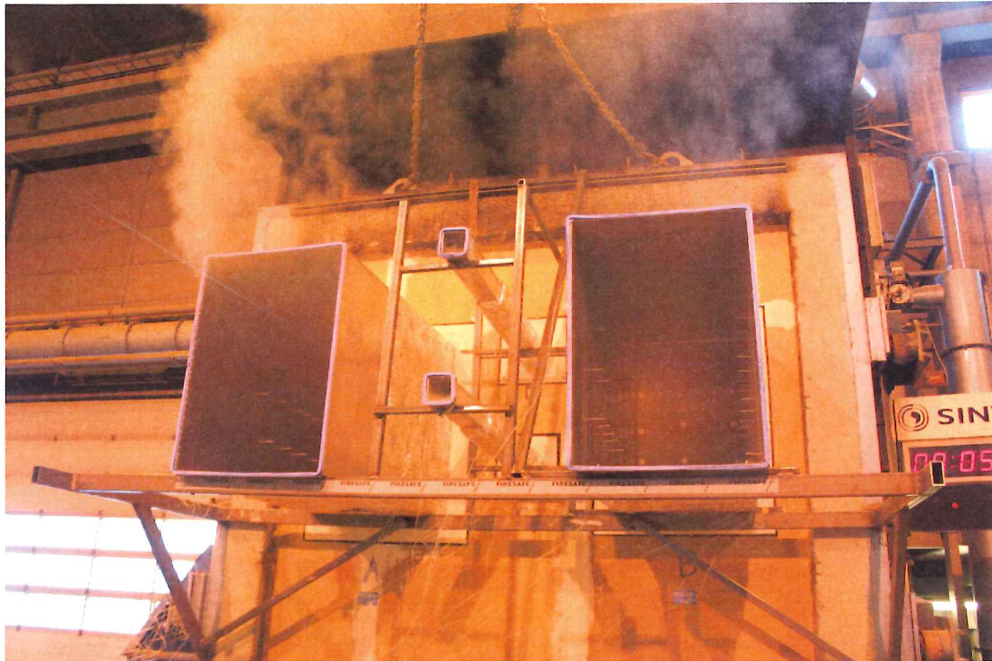
Photo 7: Smoke comes out of ducts after 8 minutes.
