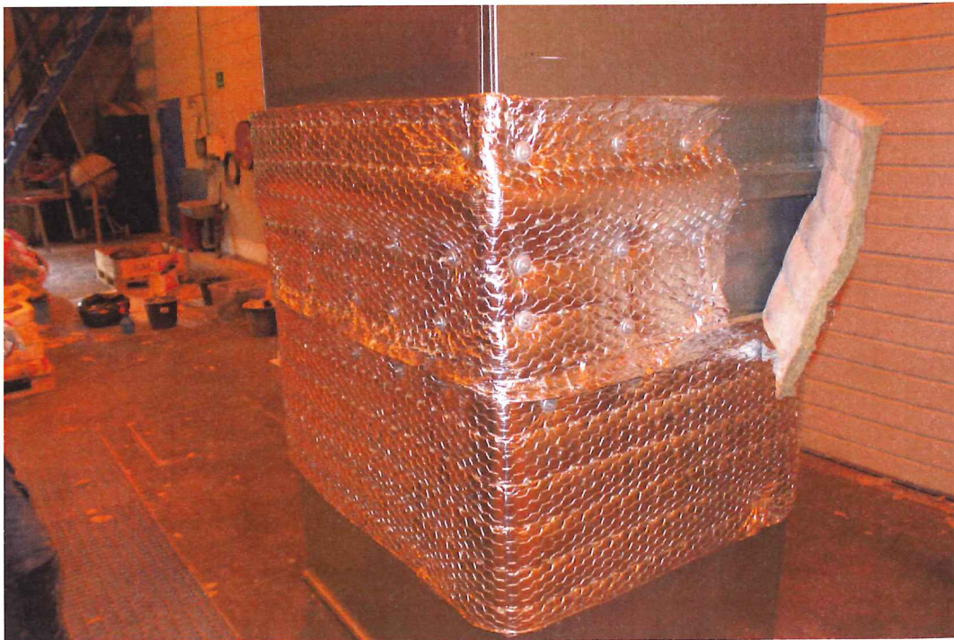
Photo 4: Duct insulation. "Paroc Wired Mat 80"
